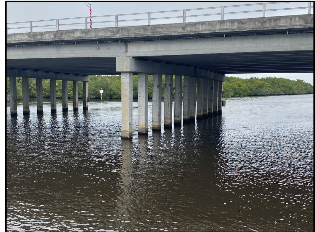
Eastern bridge section of SR 716/Southeast Port St. Lucie Boulevard looking north (pre-construction)
